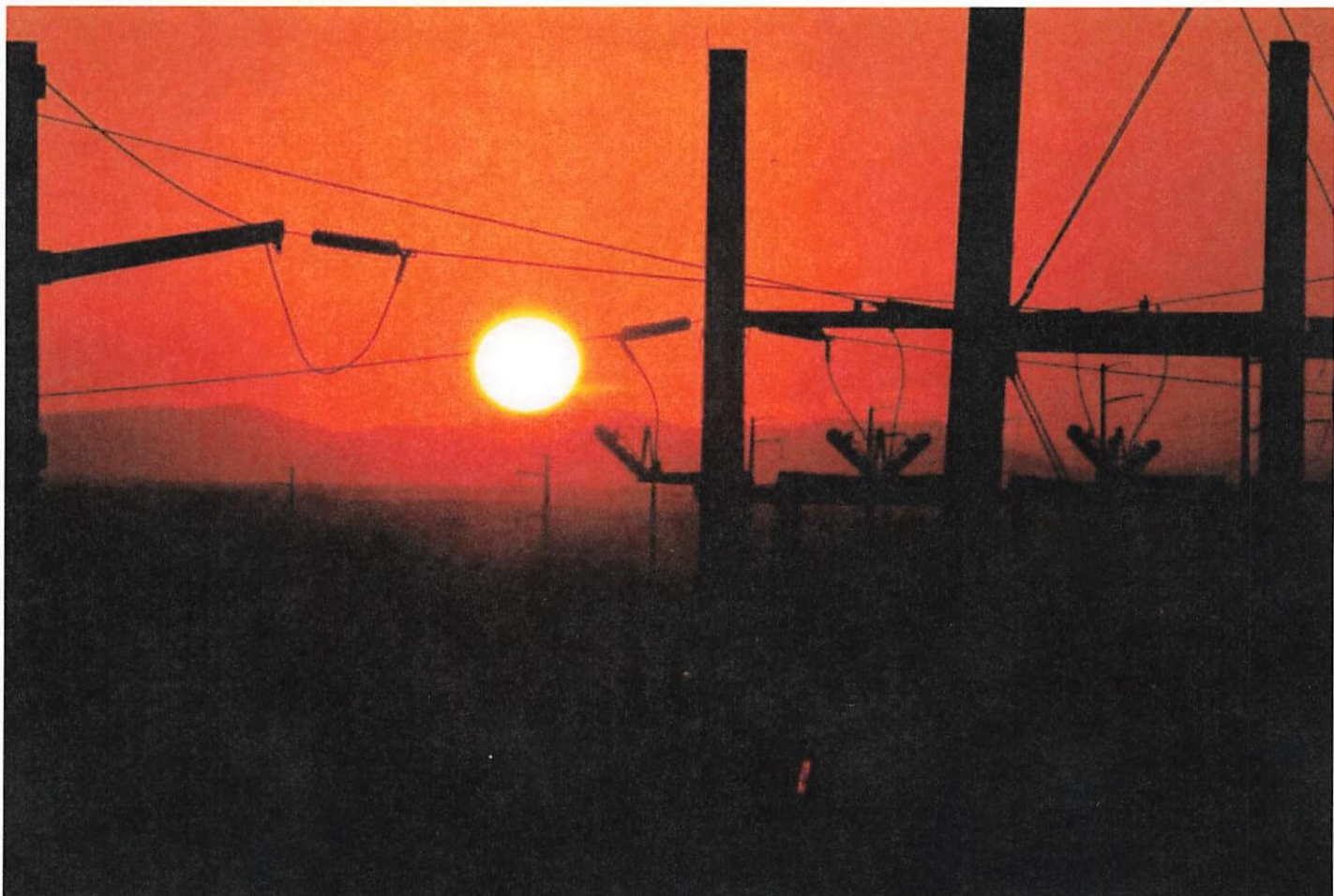
Electrical infrastructure at sunset.
