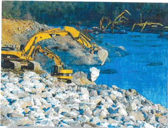
RSP - Oroville Dam Spillway Emergency Response
