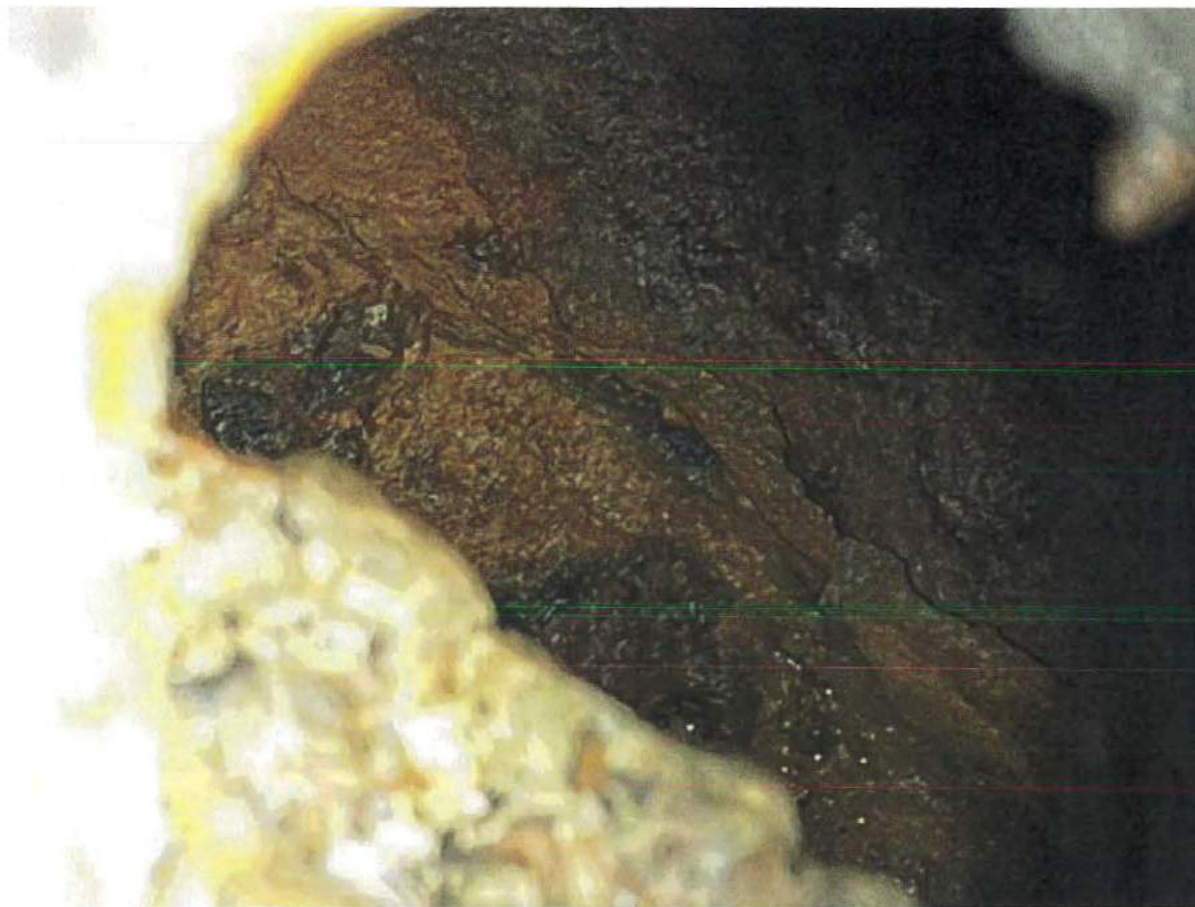
View of debris in cavity below 42" piston (12).
